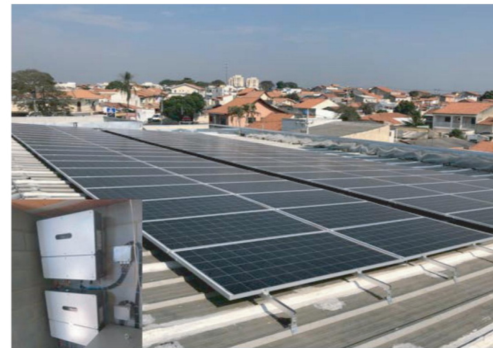
Brazil 500kW Rooftop Project
