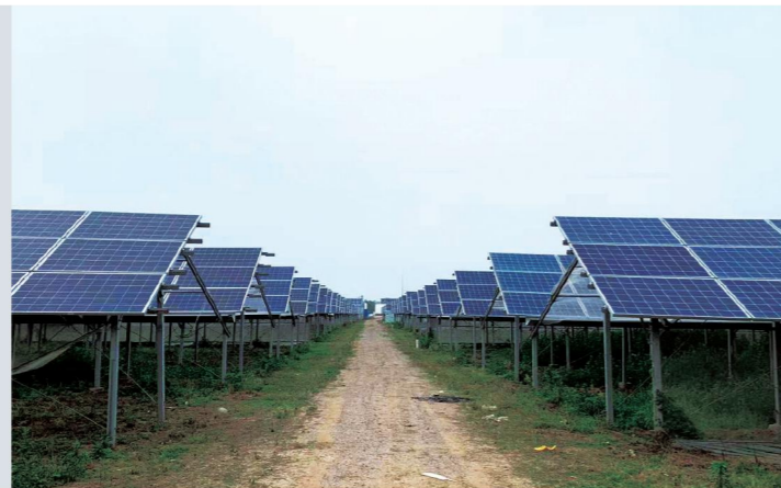
Solar Renewable Project in Anqiu
