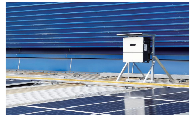
12MW Dalian Roof-top PV Project in China
