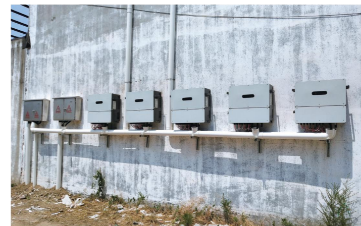
Rooftop PV Project in Shandong
