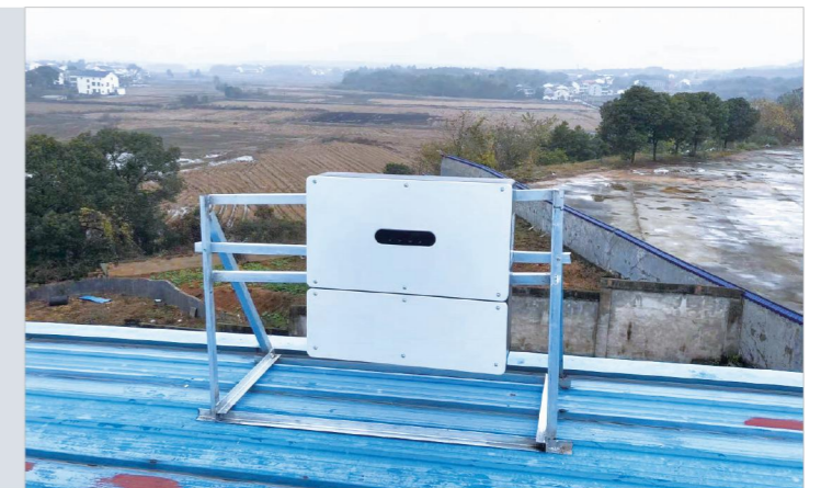
Roof-top PV Project in Hunan China
